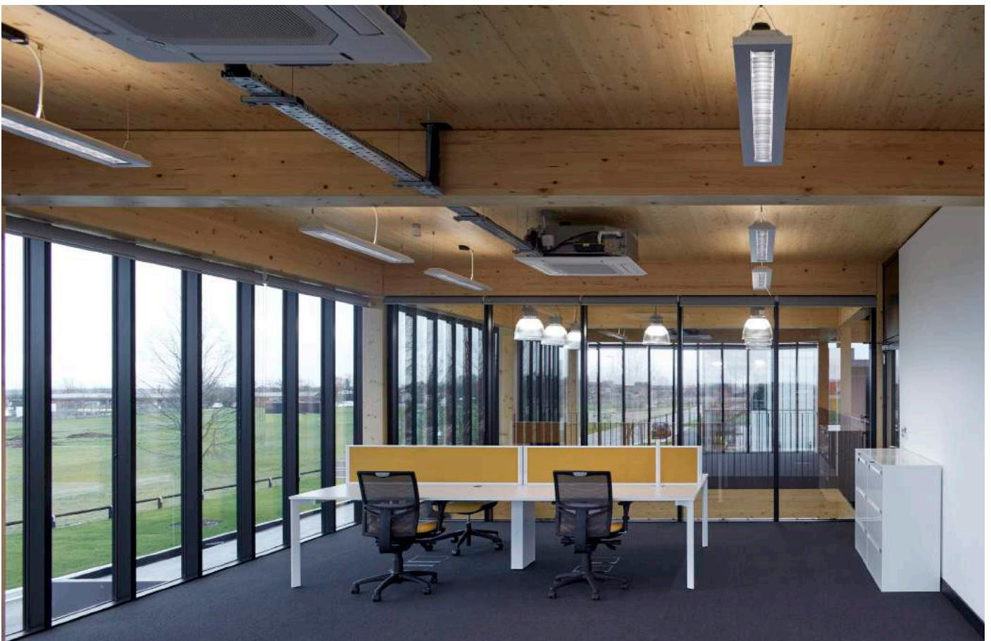
Urban&Civic office space at Alconbury Weald Club showing cassette units fed from raised floor zone above
